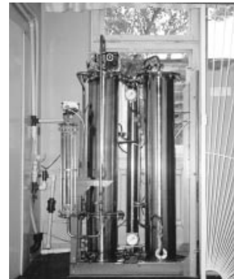
The Center for Water Resources supervised the development and installation of this water purification system in Okhmatdet Children's Hospital, largest in the Ukraine. Its modular design allows for varying levels of purification depending on the nature of water use. The Center has entered into a contract to supply 40 systems in Ukrainian hospitals and schools.
