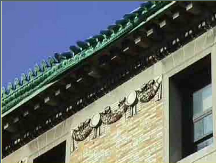
BXCC: damaged cornice of Philosophy Hall
