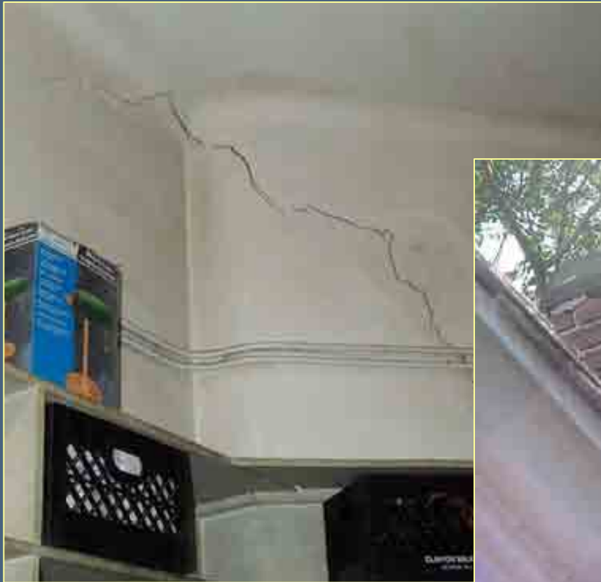
Queens College: cracks in structure of Jefferson Hall
