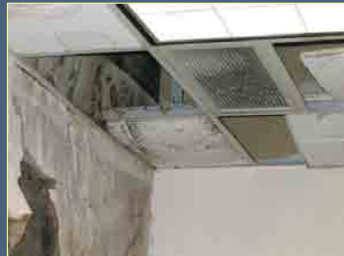
NYCC Tech: water damage in Student Lounge in "G" Bldg
