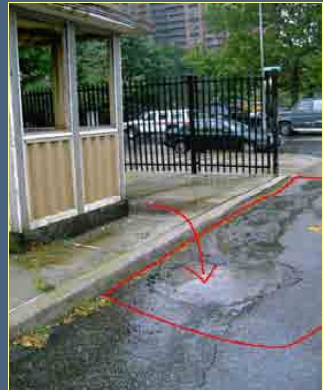
Medgar Evers: potholes in parking lot
