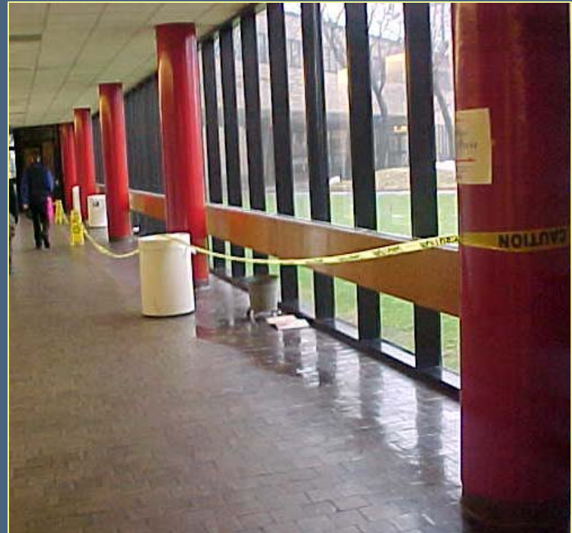
Kingsborough CC: water infiltration in passageway of "P" bldg
