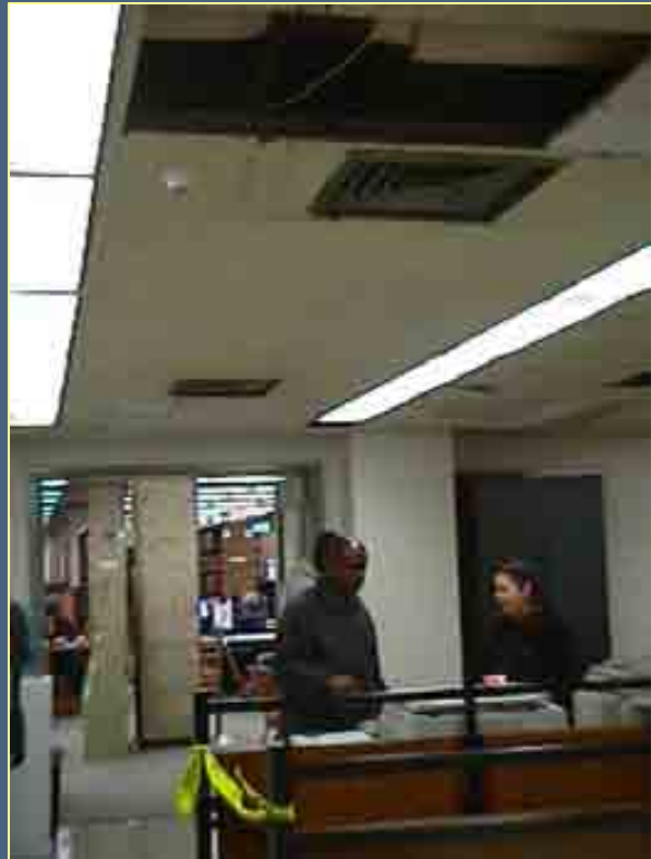
BXCC: leaks in library ceiling
